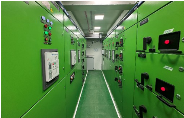
Philippines | MNL1 Data Center Project
